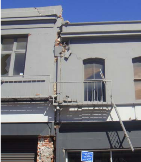
Figure 6: Pounding-induced damage of buildings in Christchurch CBD 3
