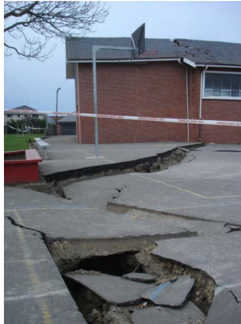
Figure 8 Lateral spread crack running through the courtyard and building at St. Paul's church, Dallington, Christchurch, New Zealand (September 2010) 6
